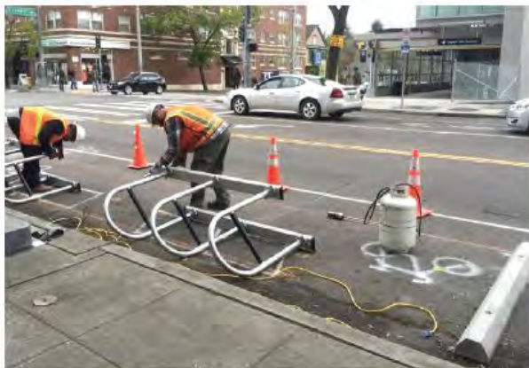
On-street bicycle corral installation at Capitol Hill Light Rail Station (Photo: SDOT)
